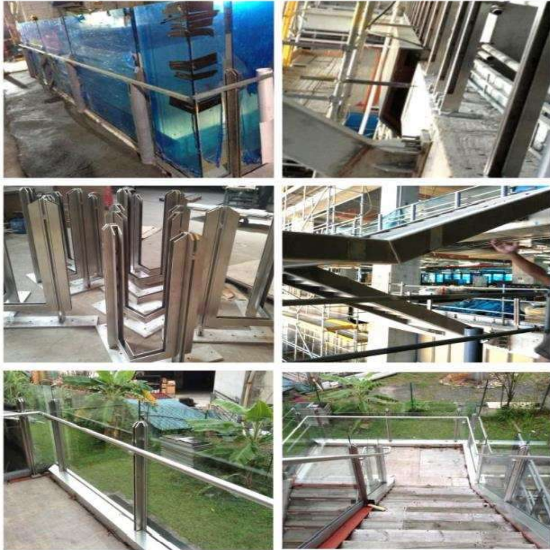
SS 316L SHOPPING MALL STAIR & RAILING SOLUTION, SINGAPORE
